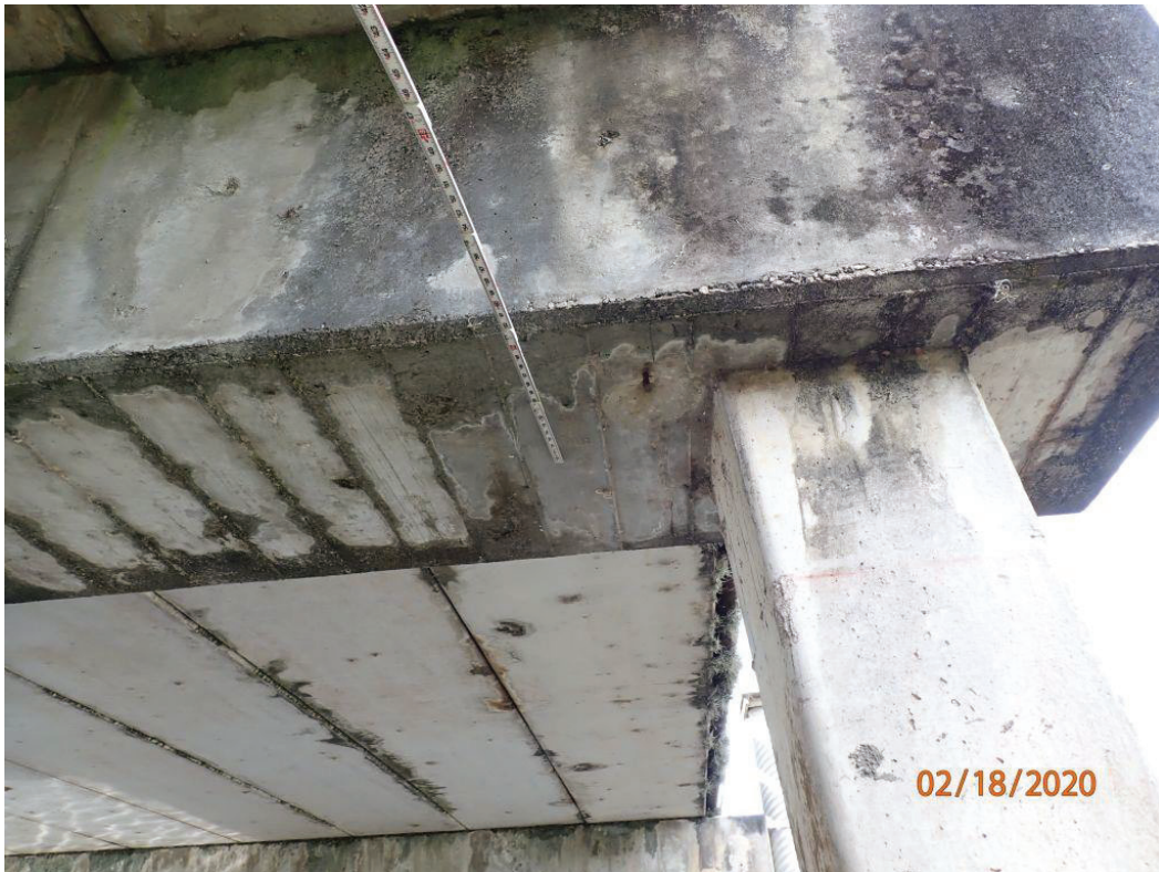
Photo 6: Element 234: Spall with exposed steel on underside of Bent 5.
