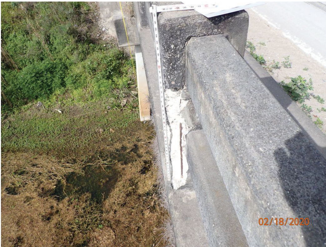
Photo 8: Element 331: Showing post spall/delamination with exposed steel.
