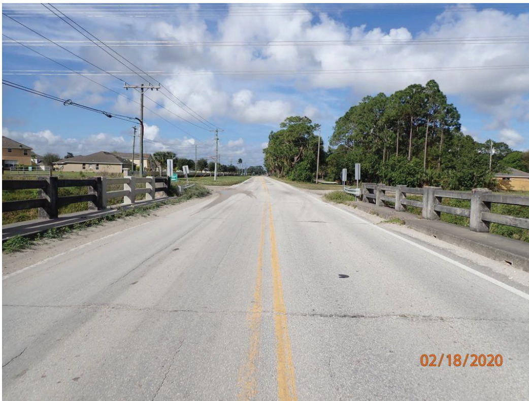
Photo 12: Inspection Notes: Faded and chipped striping on bridge.
