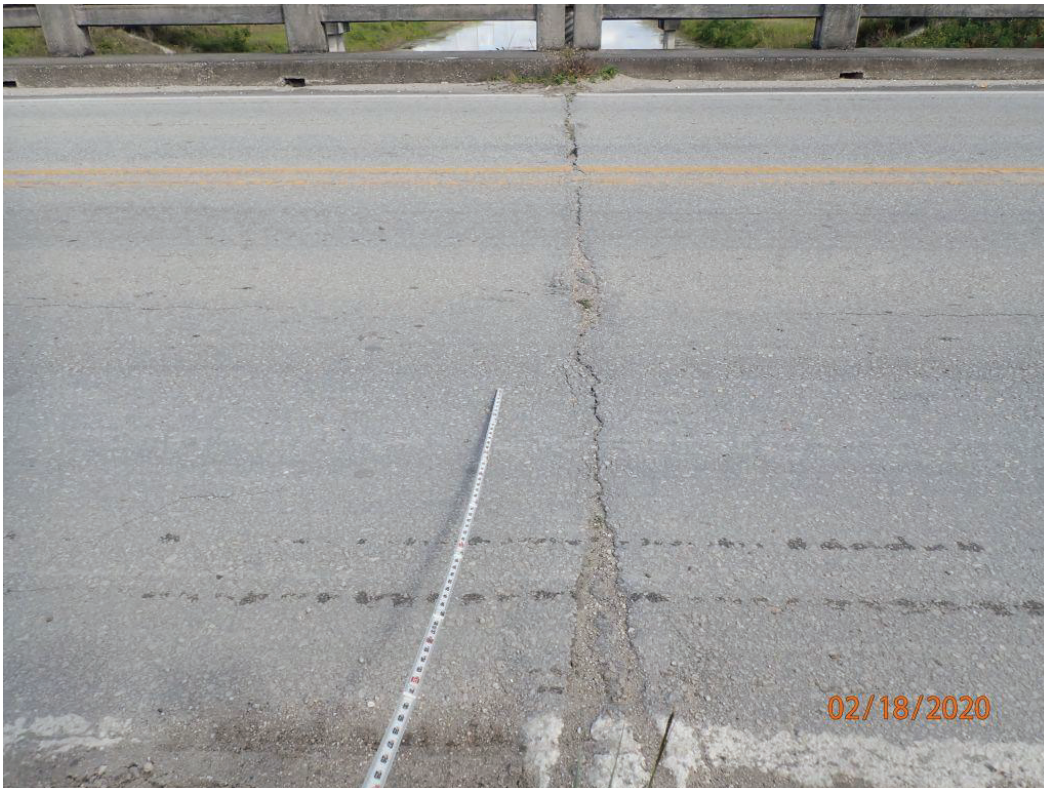
Photo 2: Element 8099: Showing transverse cracks with potholes in AC overlay at Bent 4.
