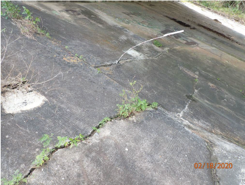
Photo 7: Element 8394: Showing northeast panel repairs and original fractures.
