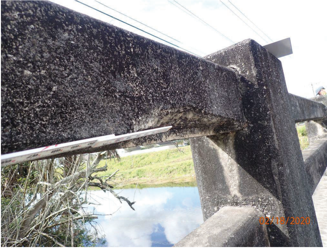
Photo 9: Element 331: Showing spall with exposed steel in bridge rail top.
