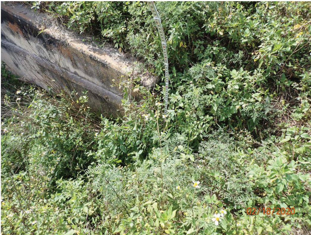
Photo 4: Element 8475: Showing northwest wingwall corner washout.
