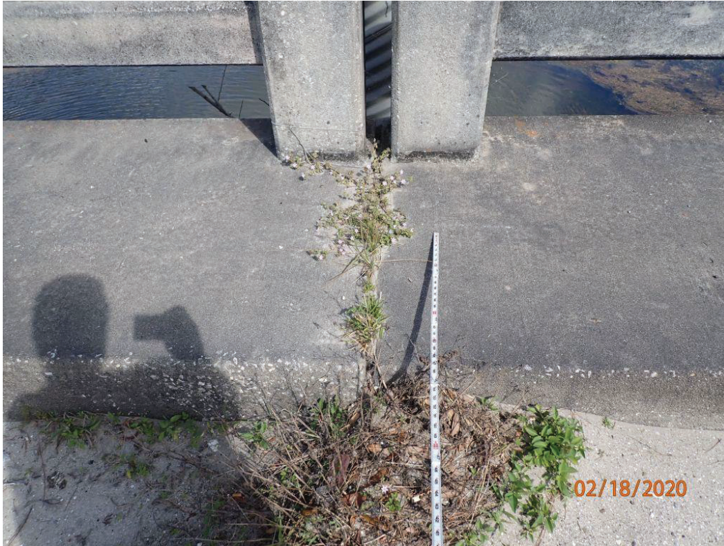
Photo 3: Element 301: Sidewalk expansion joint deteriorated sealant, dirt and debris
