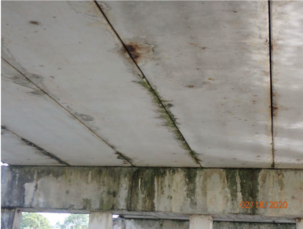
Photo 1: Element 8099: Showing leaking and staining in the slab unit joints.
