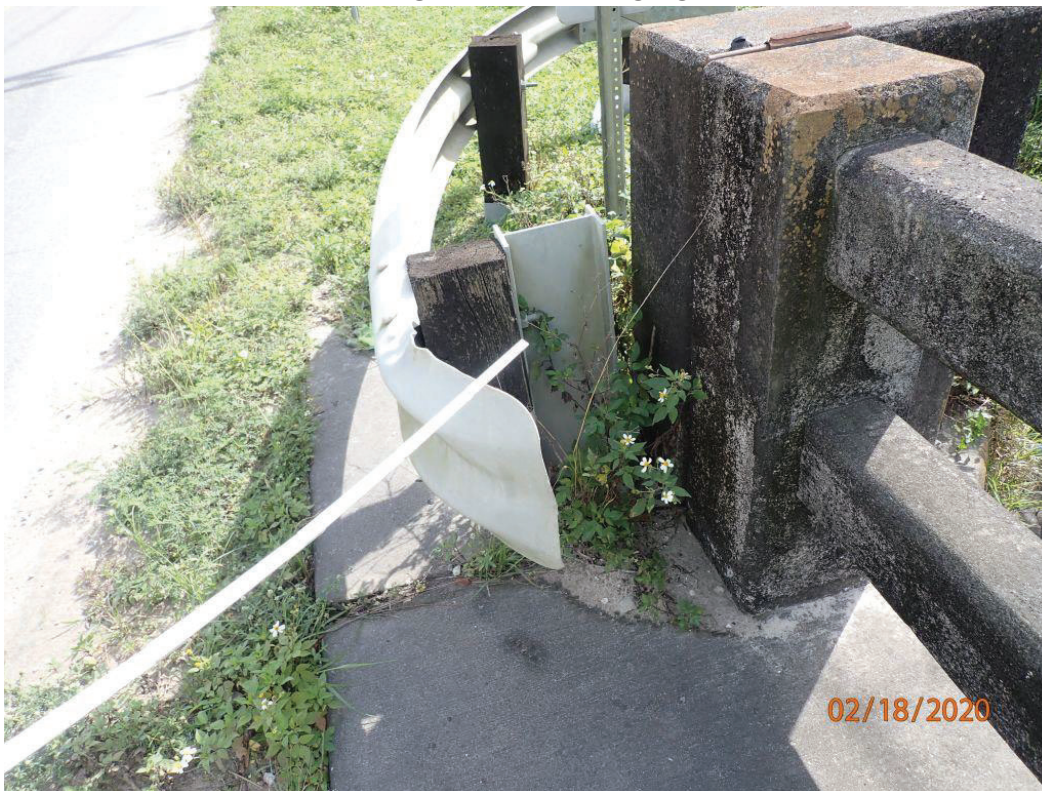
Photo 11: Inspection Notes: Showing approach guardrail not attached to structure.
