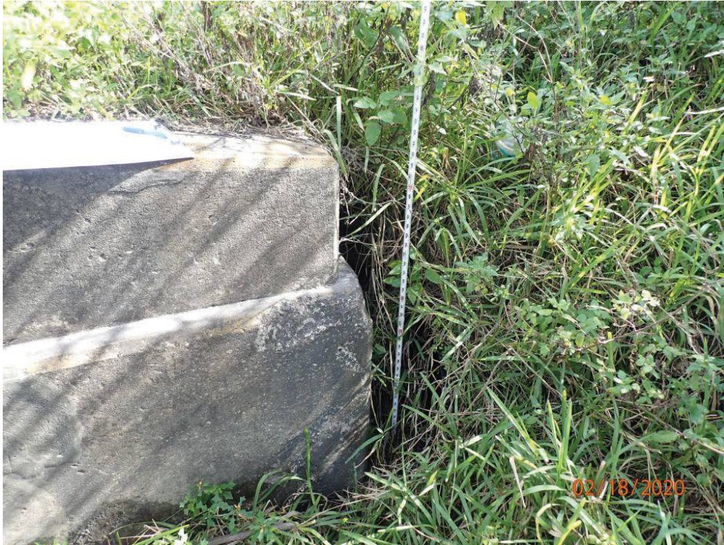
Photo 5: Element 8475: Showing southeast wingwall corner washout.
