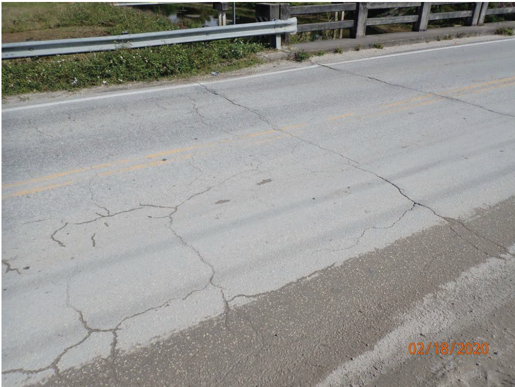
Photo 10: Inspection Notes: Showing cracks with light dirt and vegetation in the approach slab/roadway transition.
